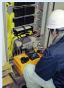
Splicing in ODF
